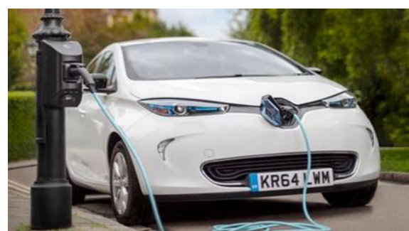
Figure 7 - Installation with EV charging device
