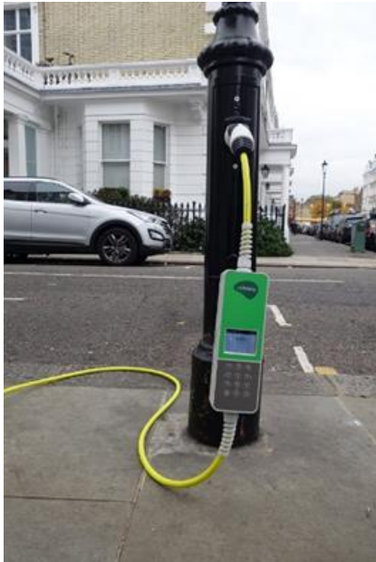
Figure 8 - Installation with the EV charging device on the cable
