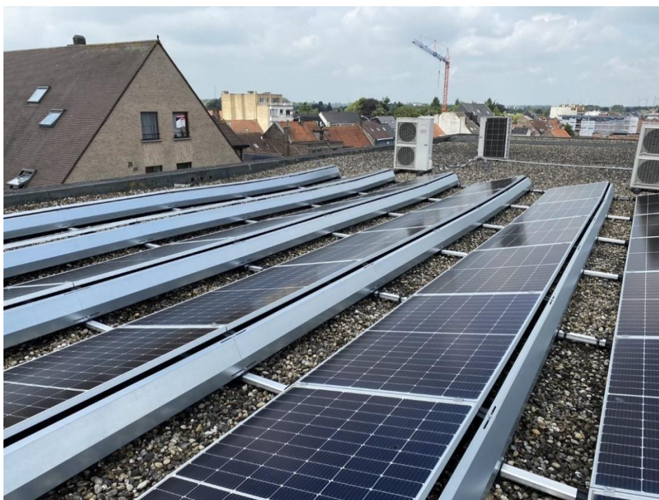
Figure 2 - Solar panels in a south-facing configuration
