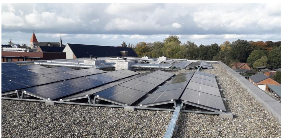
Figure 1 - Solar panels in an east-west configuration
