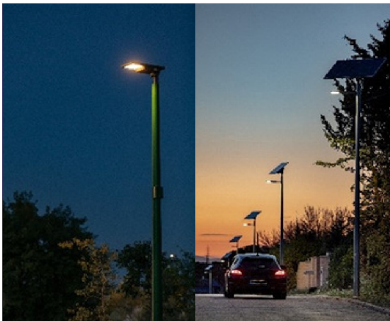
Luminaires by night
