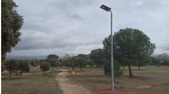
All in one luminaire in public park
