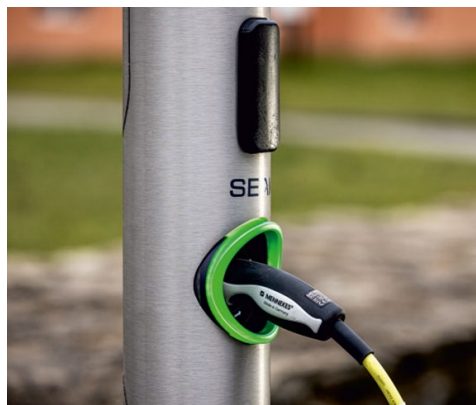
Figure 12 - Seak Solution for EV Charging
