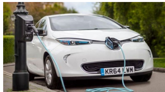
Figure 7 - Installation with EV charging device
