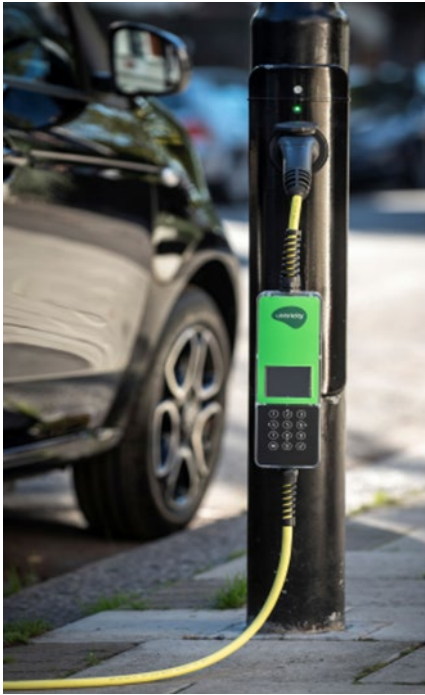
Figure 9 - Lucy Zodion Trojan Midi with 32 A disconnecter
