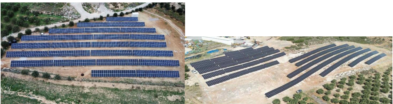
Top views of the first two photovoltaic parks of MEC, of 405 kW and 1 MW nominal capacity.
